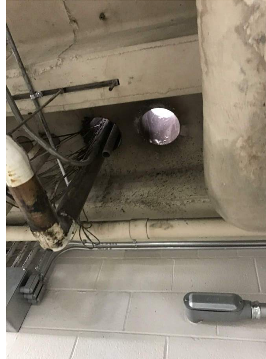
EXISTING SLEEVE THRU CONC CEILING/FLOOR FOR NEW SANITARY LINE ROUTING. FILL ANNULAR SPACE AFTER PLUMBING WORK IS COMPLETED WITH FIRE CAULKING MATERIAL.
