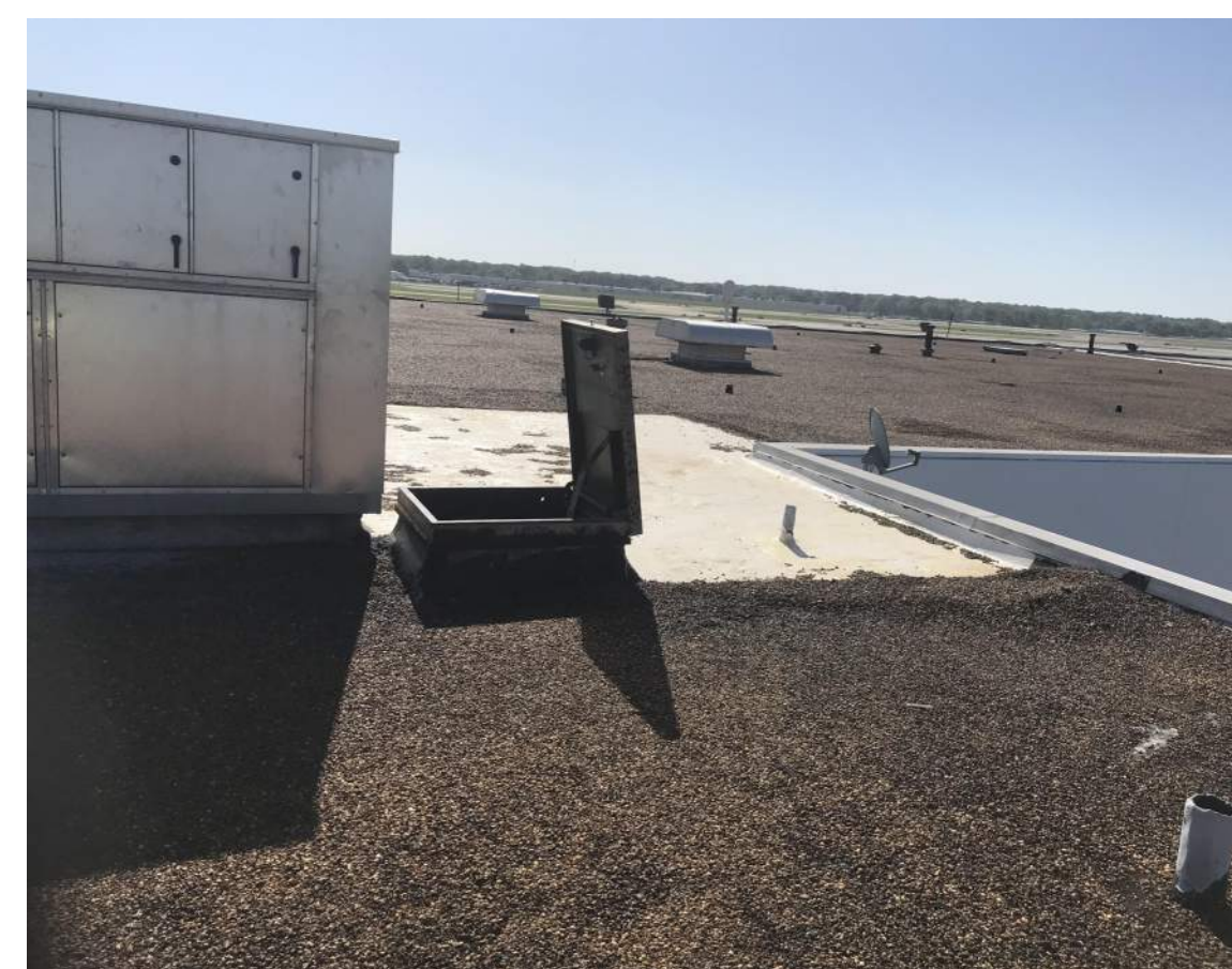
PHOTO 5 THE CONTRACTOR SHALL REMOVE ANY LOOSE PEA GRAVEL REMAINED ON THE ROOF BEFORE INSTALLATION OF NEW TPO ROOFING SYSTEM. GC TO PROVIDE AND INSTALL NEW SAFETY RAIL AND GATE ON THE EXISTING ROOF HATCH FOR FALL PROTECTION.
