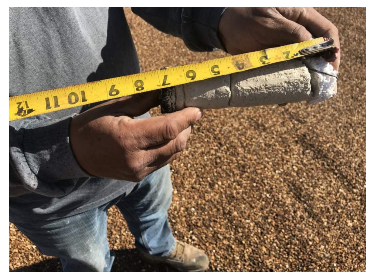
PHOTO 2 THE EXISTING ROOF IS ABOUT 4 1/2" THICK TO THE METAL DECK. THE EXISTING SYSTEM CONSISTS OF AVERAGE OF 1" WHITE EXPANDED POLYSTYRENE FOAM BOARD UNDER APPROXIMATELY 4"-7" THICK OF LIGHT WEIGHT INSULATED CONCRETE UNDER THE ASPHALT BUILD-UP ROOF AND PEA GRAVEL. THICKNESS OF EXISTING LIGHT WEIGHT INSULATED CONCRETE SUBSTRATE VARIES IN ORDER TO CREATE THE IN-PLACE SLOPE FOR DRAINAGE. REMOVE PEA GRAVEL WHEREVER FEASIBLE FOR SOUND SECUREMENT OF COVER BOARD.
