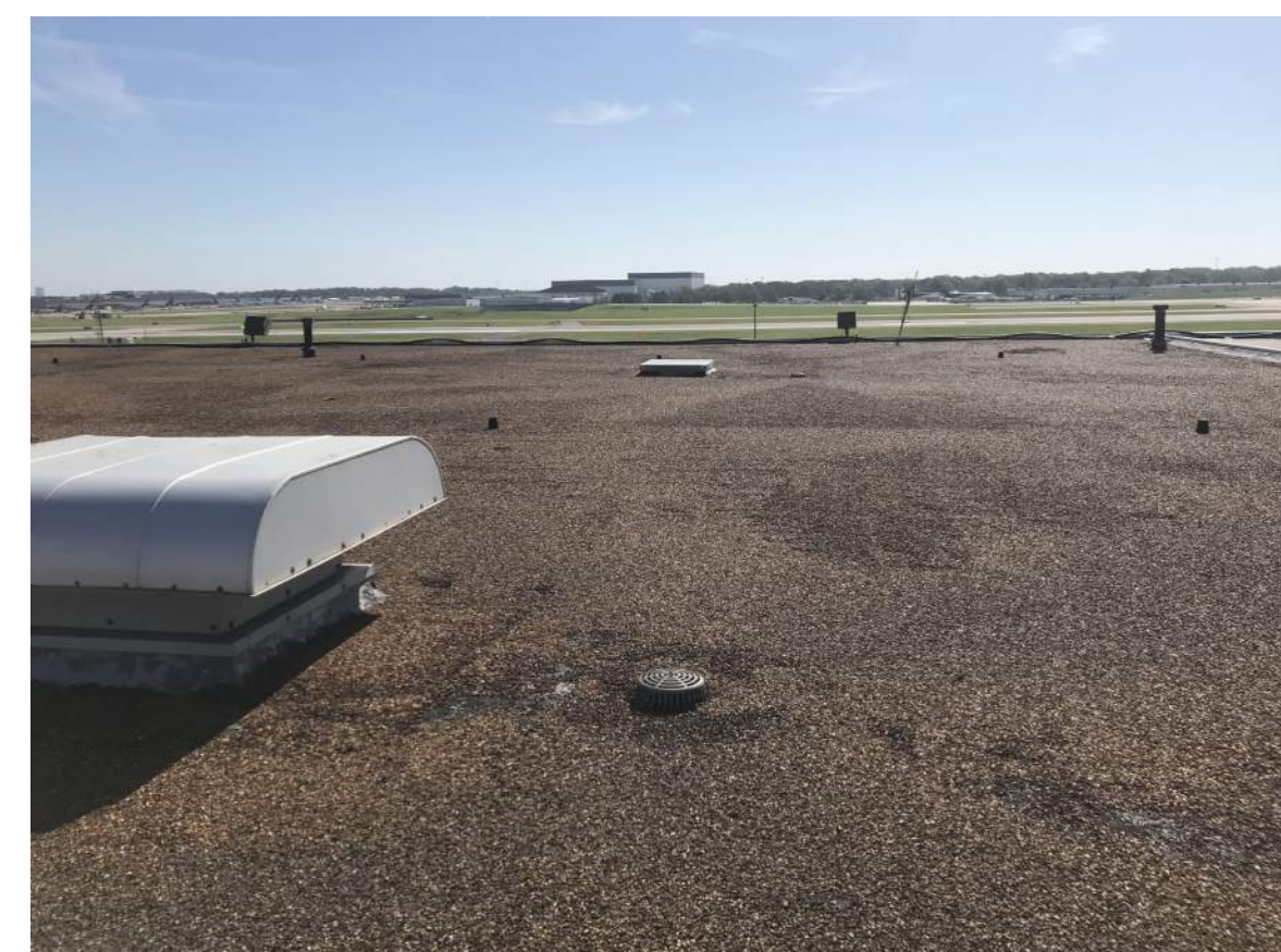
PHOTO 1 SUMP DRAIN AREA FOR PROPER DRAINAGE. INSTALL FLASHING AND RTU METAL AROUND EXISTING ROOF EQUIPMENT. MEMBRANE TO BE FULL ADHERED TO NEWLY MECHANICAL ATTACHED HIGH DENSITY POLYISOCYANURATE RIGID COVER BOARD INSULATION. CORRECT ANY AREA AS NEEDED TO SLOPE TOWARD EXISTING ROOF DRAINS. REF ROOF PLAN.
