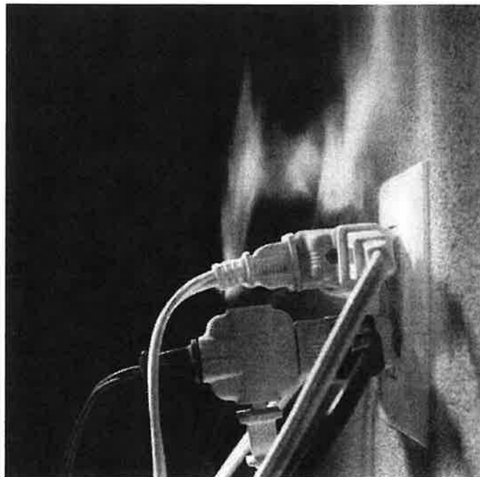
Figure 2 Example of an overloaded electrical outlet
