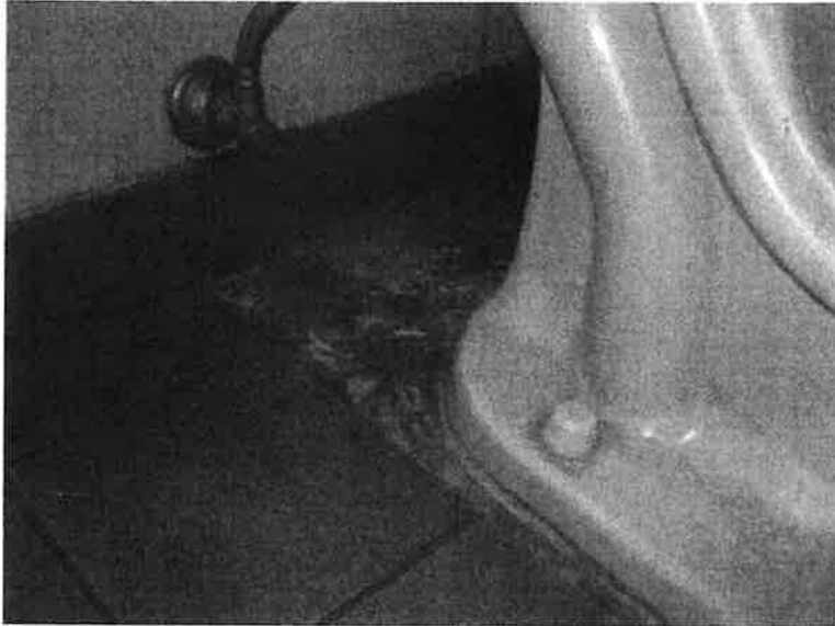
Figure 32 Dirt behind a Toilet
