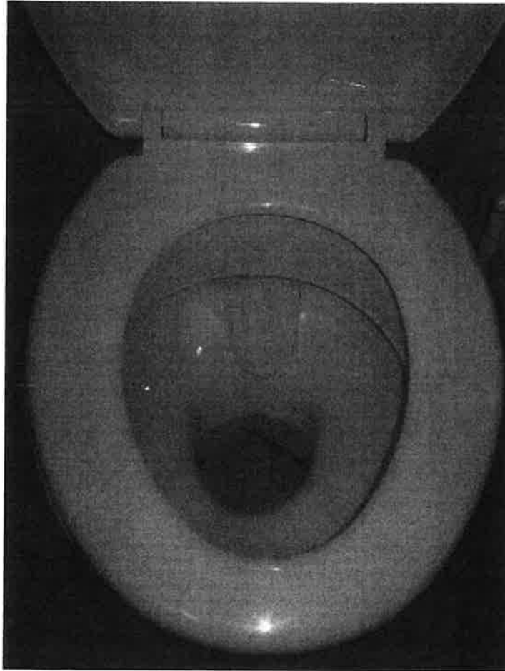
Figure 45 Dirty toilet bowl and hole at bottom
