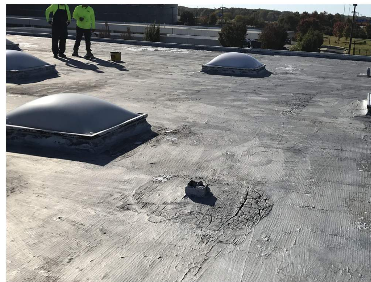
PHOTO 12 SAFETY HARNESS ANCHOR POINTS SHALL REMAIN AS IS. PROVIDE SEALANT POCKET TO ENSURE THE AREA IS WATER TIGHT
