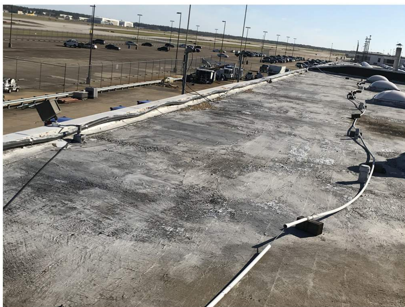
PHOTO 11 COORDINATE WITH AIRPORT AUTHORITY ON PROPER REINSTALLATION OR REMOVAL OF THE CABLING LEFT ON THE ROOF TOP.
