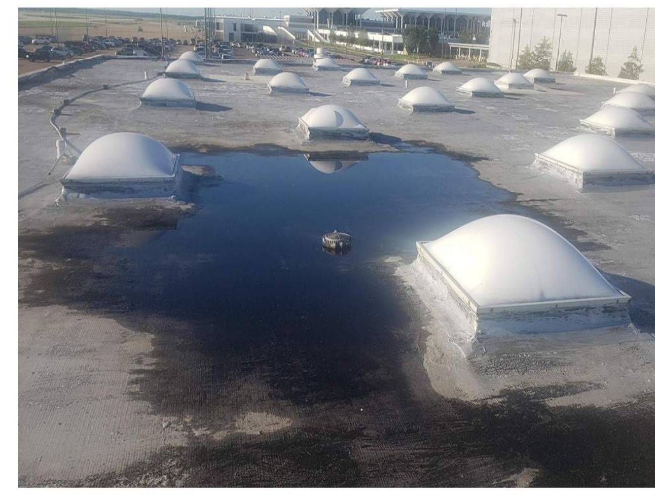
PHOTO 13 AREA OF PONDING SHALL BE CORRECTED TO ALLOW PROPER DRAINAGE FLOW. CLEAN THE DRAIN LINE AS NEEDED TO ENSURE PROPER FLOW. ALL EXISTING AREA DRAIN SHALL BE REPLACED WITH NEW DRAIN OF SAME SIZE AND RECONNECT SECURELY FOR PROPER FLOW.
