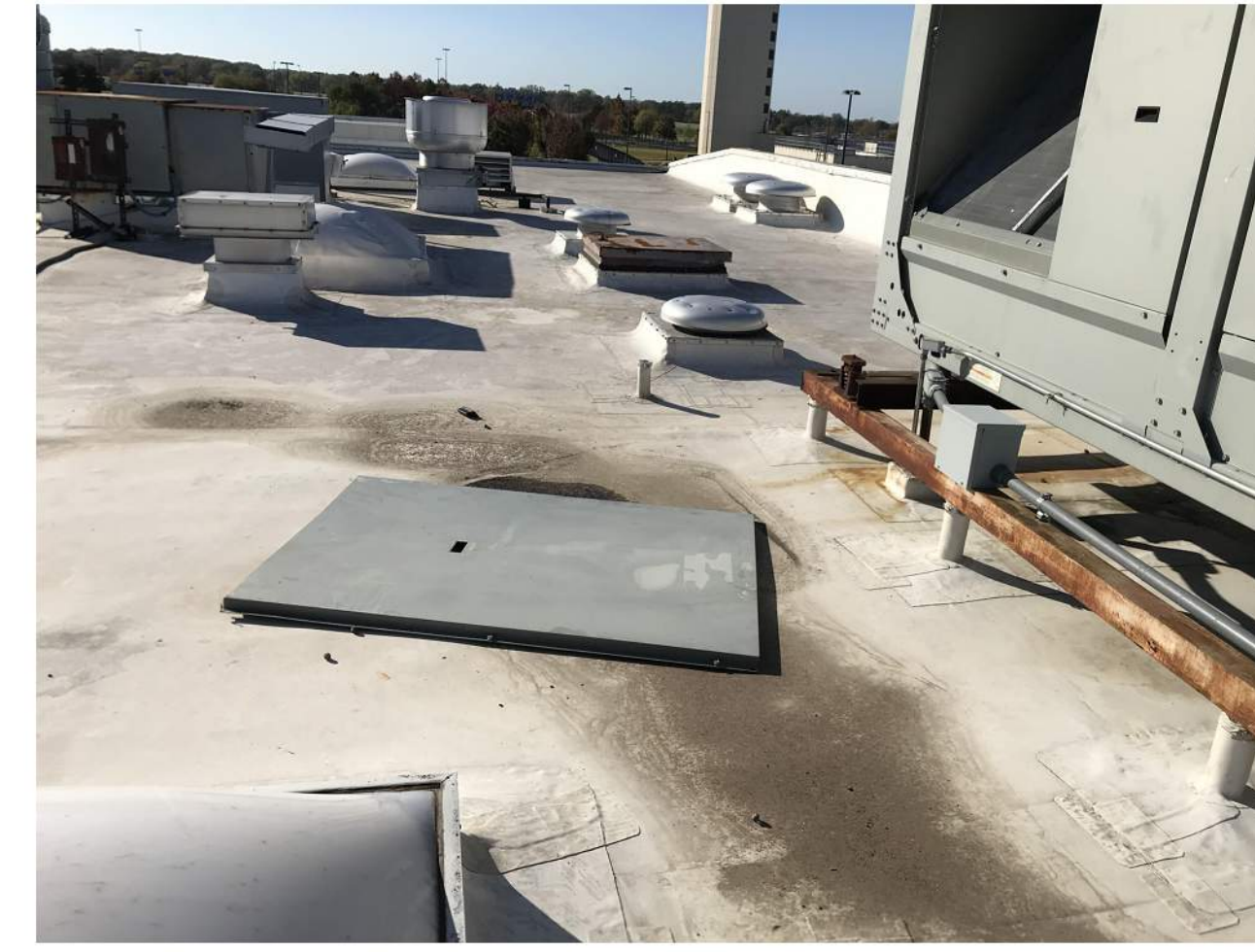
PHOTO 9 TPO ROOFING TO REMAIN AS IS IN THE MIDDLE PORTION OF THE BUILDING THAT WAS RECENTLY INSTALLED. ALL SKYLIGHT AT THESE AREA TO BE REMOVED ALSO AND BE COVERED WITH INSULATION OVER METAL DECKING TO SPAN OVER THE EXISTING CURB. SLOPE TOP TO DRAIN SO THAT WATER PONDING WOULD NOT BE POSSIBLE.
