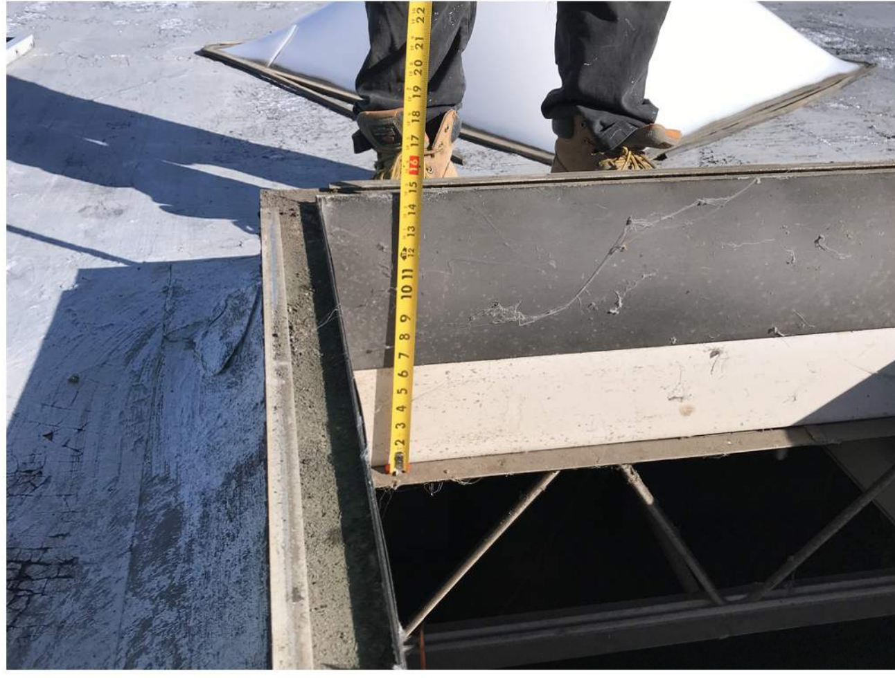
PHOTO 7 ABOVE THE JOIST IS 6" OF COMPOSITE CONSISTS OF LIGHT WEIGHT INSULATED CONCRETE ON CORRUGATED METAL DECKING. THE OVERALL HEIGHT OF THE SKYLIGHT ON THE CONCRETE IS ABOUT 9 INCHES. THE WIDTH OF FLANGES IS ABOUT 2 1/4 INCHES
