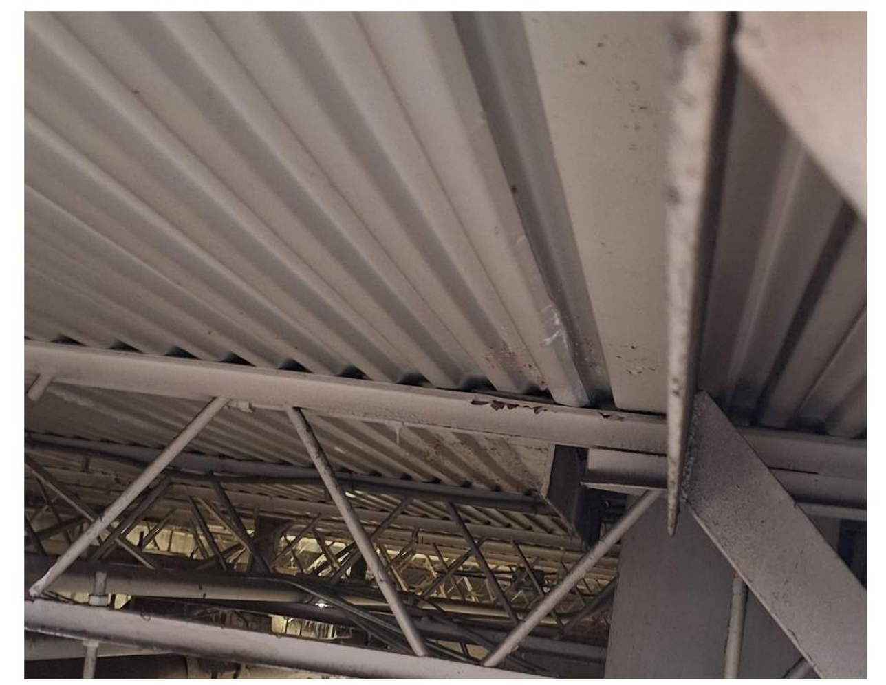
PHOTO 3 EXAMPLE OF EXISTING METAL DECKING UNDER THE LIGHT WEIGHT CONCRETE. CONTRACTOR SHALL FIELD VERIFY CONDITION OF ALL AREAS WITHIN THE PROJECT SCOPE.
