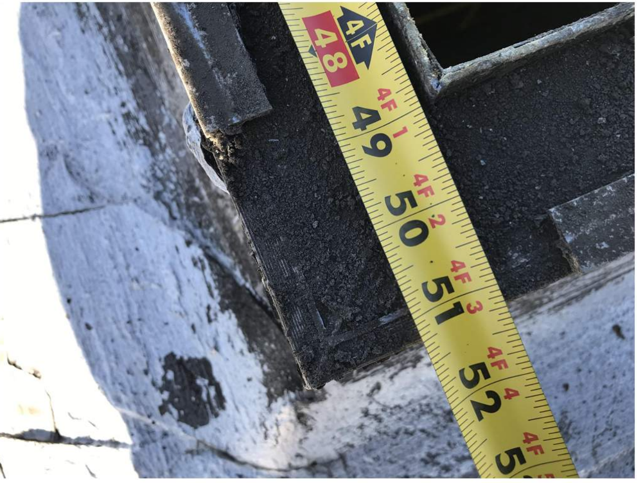
PHOTO 6 EXISTING DIMENSION OF EDGE TO EDGE OF THE DIMENSION OF THE SKYLIGHT CURB TO BE 51 1/4" BY 51 1/4"...THE INSIDE CLEARANCE IS APPROXIMATELY 48 1/2" X 48 1/2"
