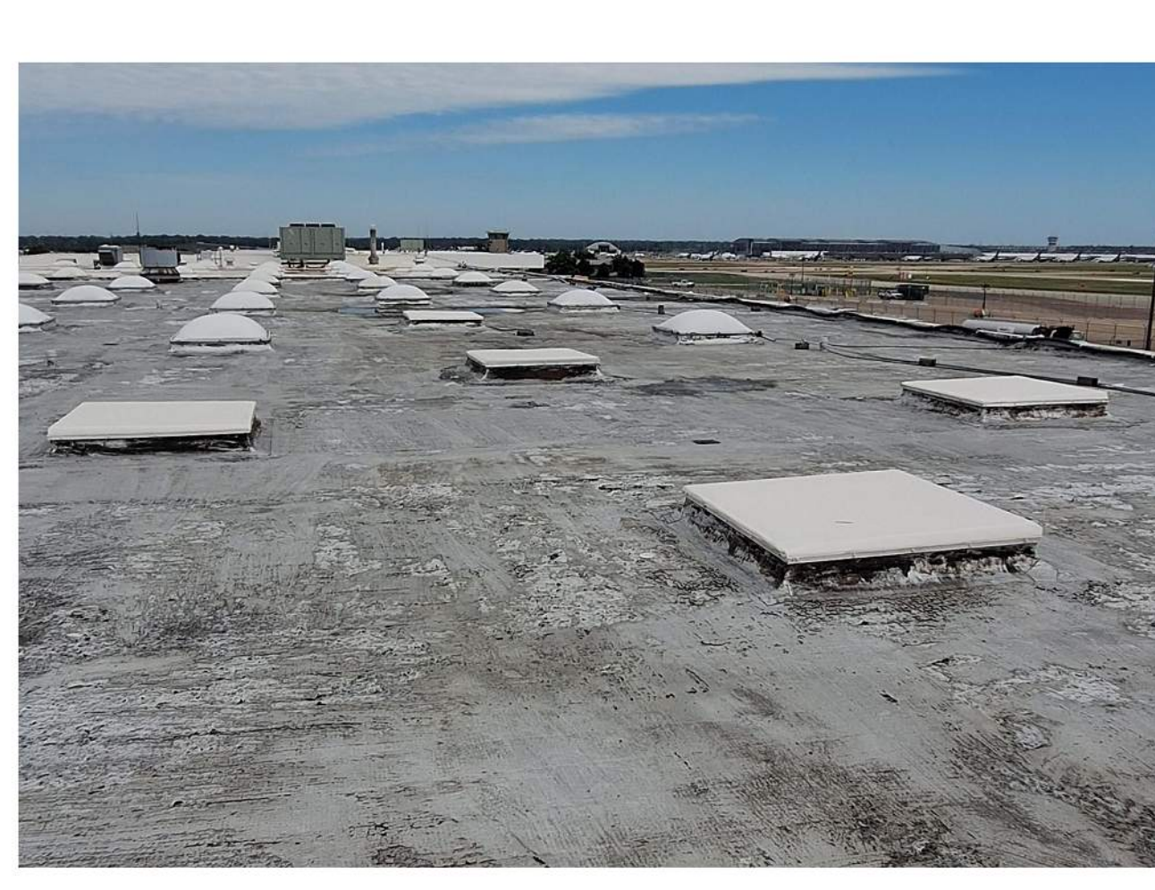
PHOTO 2 ALL REMAINING SKYLIGHTS SHALL BE REMOVED FOR ROOF RECOVERING. PORTION OF EXISTING SKYLIGHT INDICATED BY YELLOW ON DRAWING BELOW HAS ALREADY BEEN REMOVED AND COVERED BY OTHERS.
