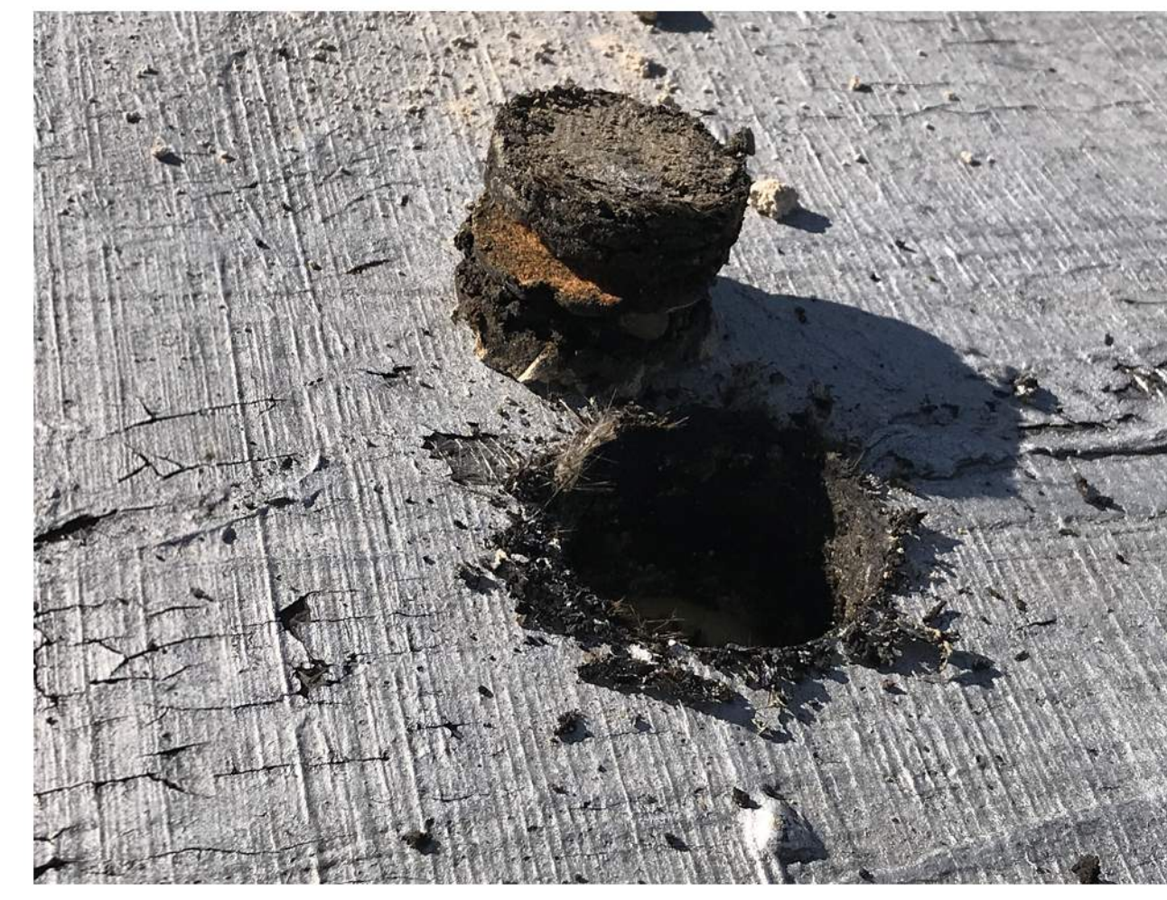
PHOTO 4 THE MAKEUP OF THE RECENT SECOND ROOF CONSISTS OF THE BUILD UP OF LAYERS OF CAPS SHEETS AND BASE SHEETS HOT MOPPED OVER FIBERBOARD THAT WAS MOPPED ONTO THE ORIGINAL PEA GRAVEL ROOF OVER LIGHT WEIGHT CONCRETE OVER ORIGINAL METAL DECKING
