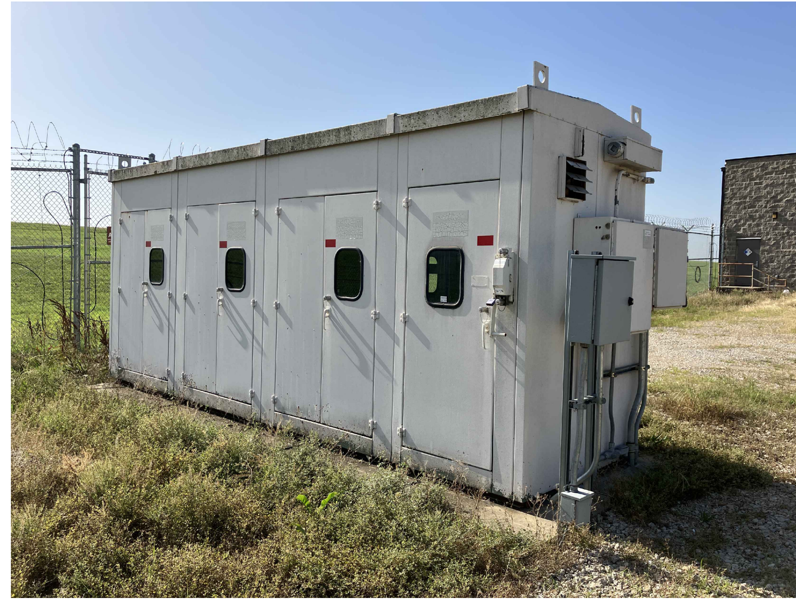
2 EXISTING CAPACITOR BANK END/FRONT VIEW SCALE: NONE
