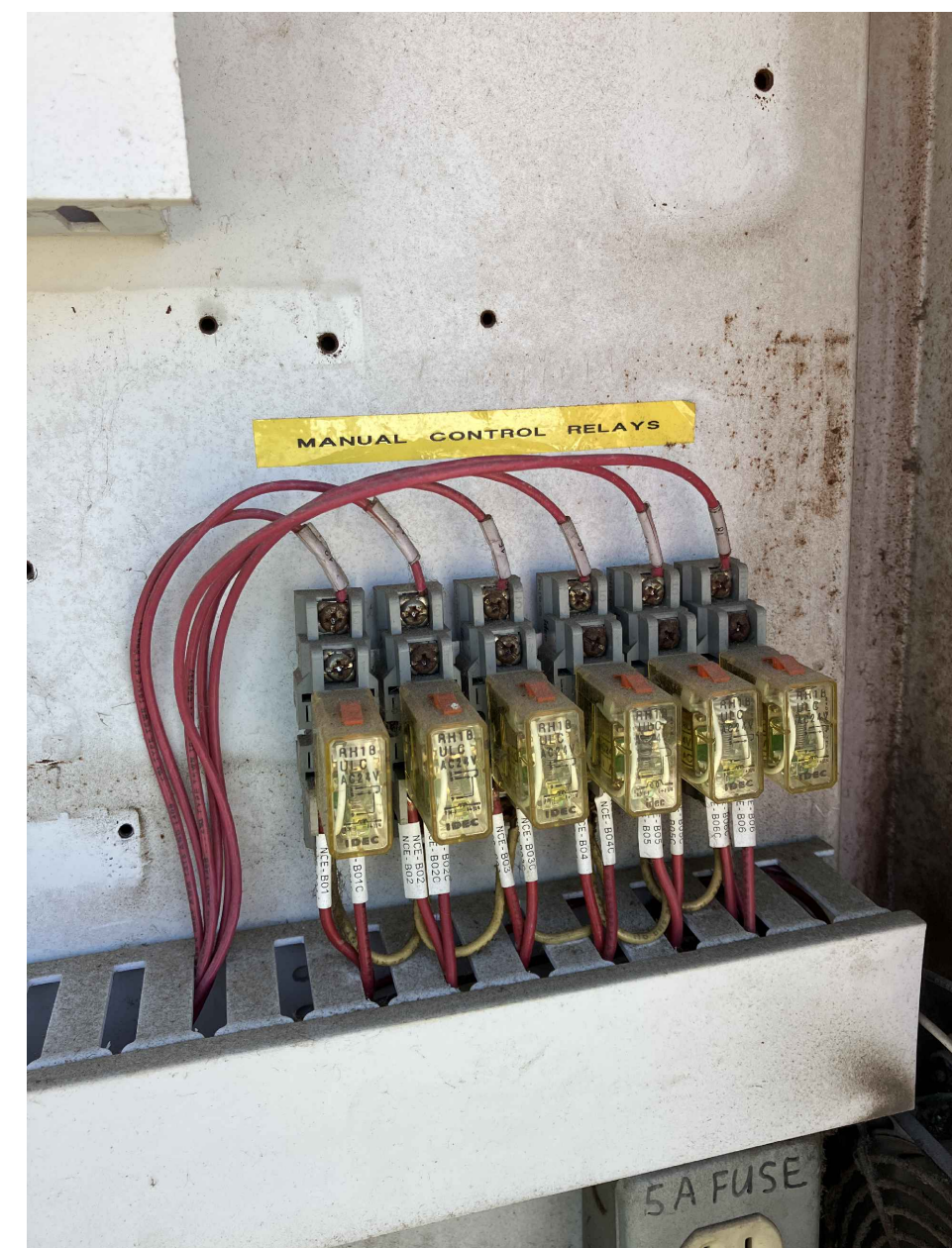
5 EXISTING JCI TERMINAL CABINET SCALE: NONE
