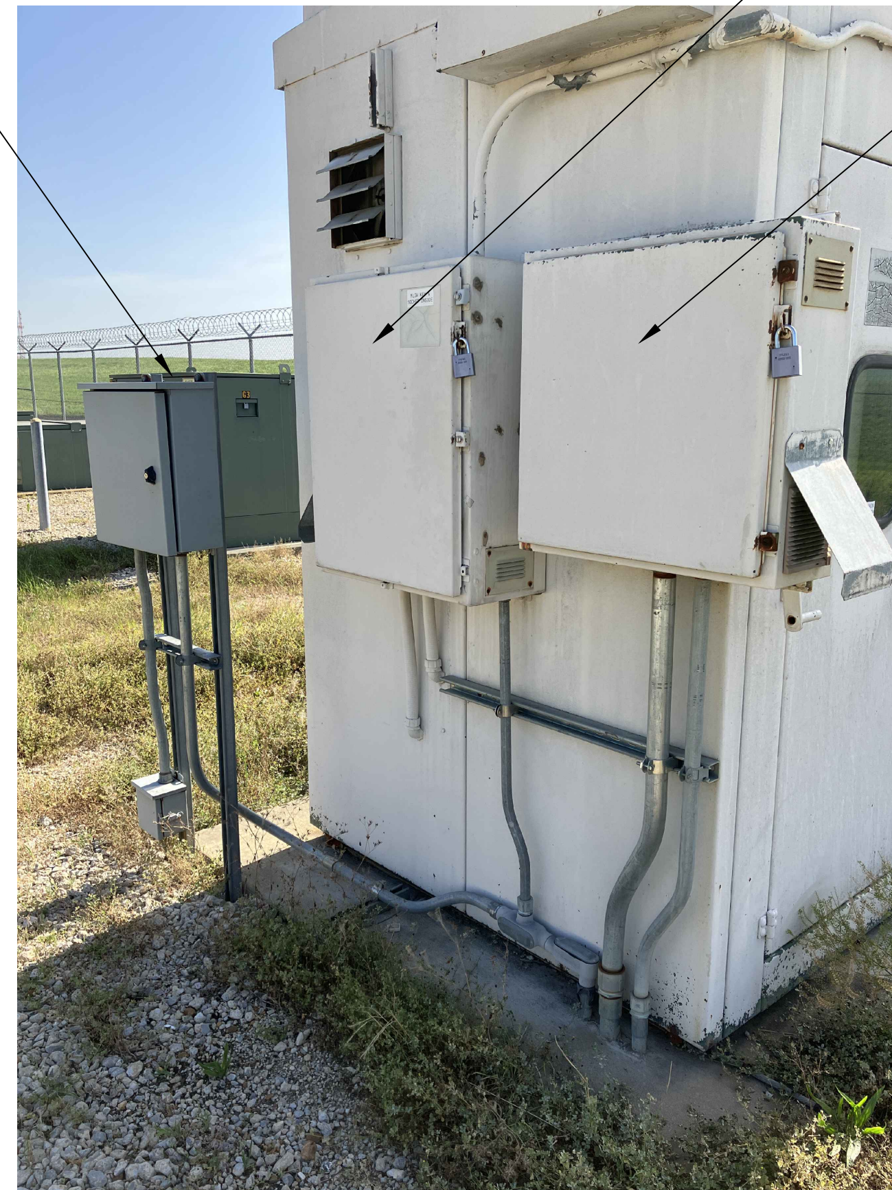
4 EXISTING CAPACITOR BANK CONTROL CABINETS W/ CONDUITS SCALE: NONE
