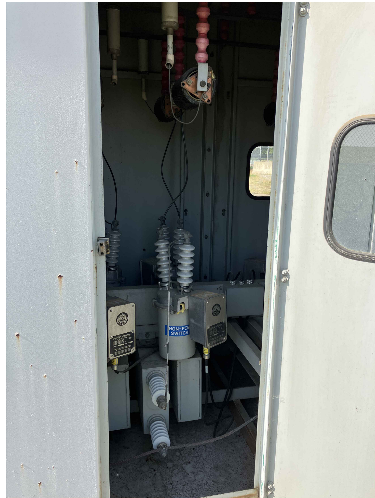
2 EXISTING CAPACITORS SCALE: NONE
