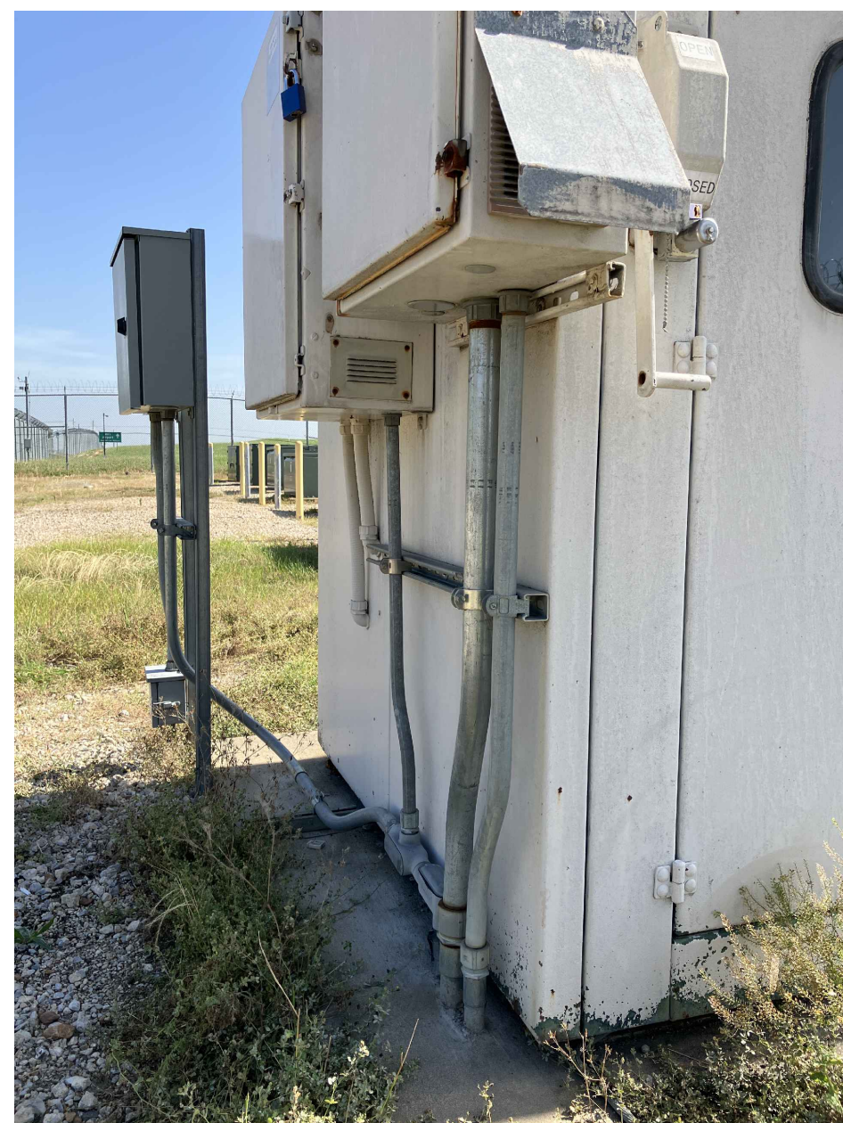
4 EXISTING CONTROLS CABINETS SCALE: NONE
