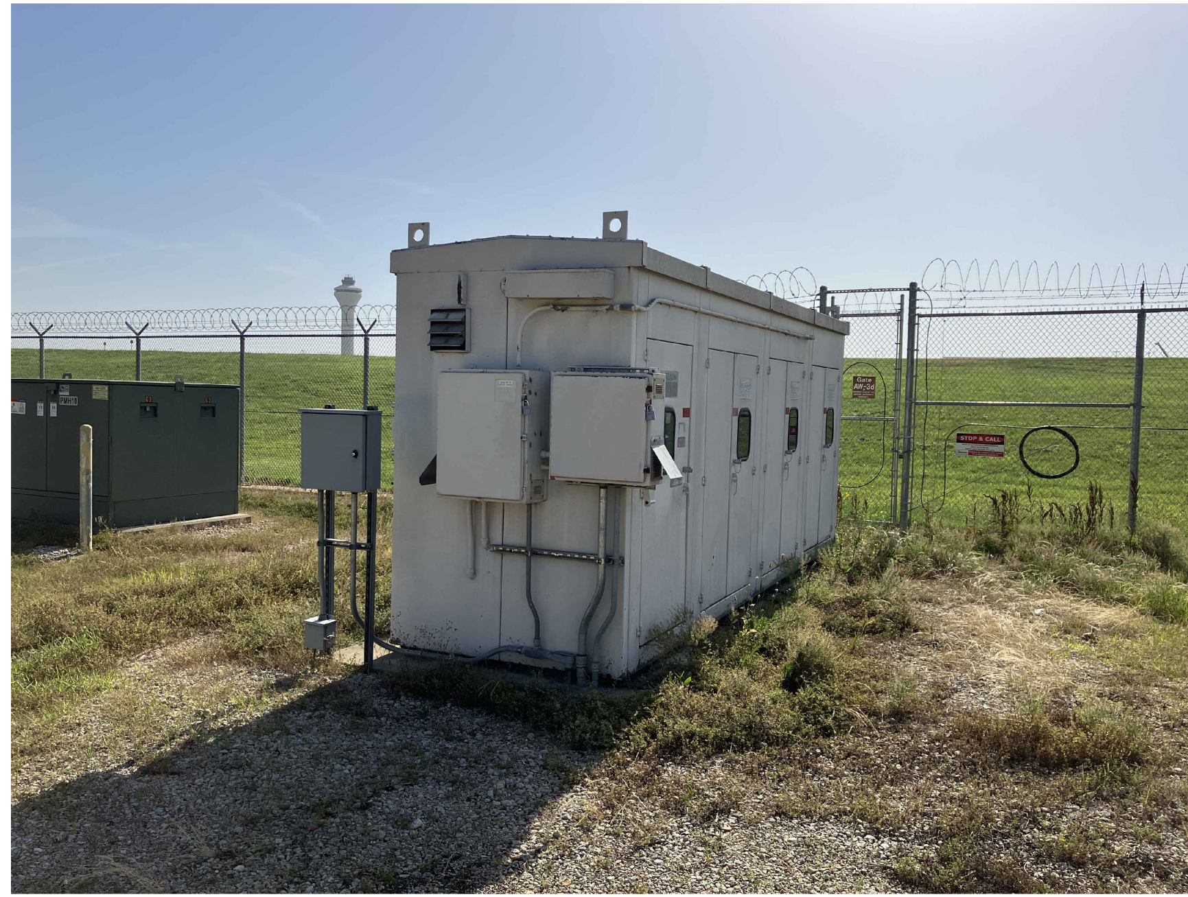
1 EXISTING CAPACITOR BANK END/FRONT VIEW SCALE: NONE
