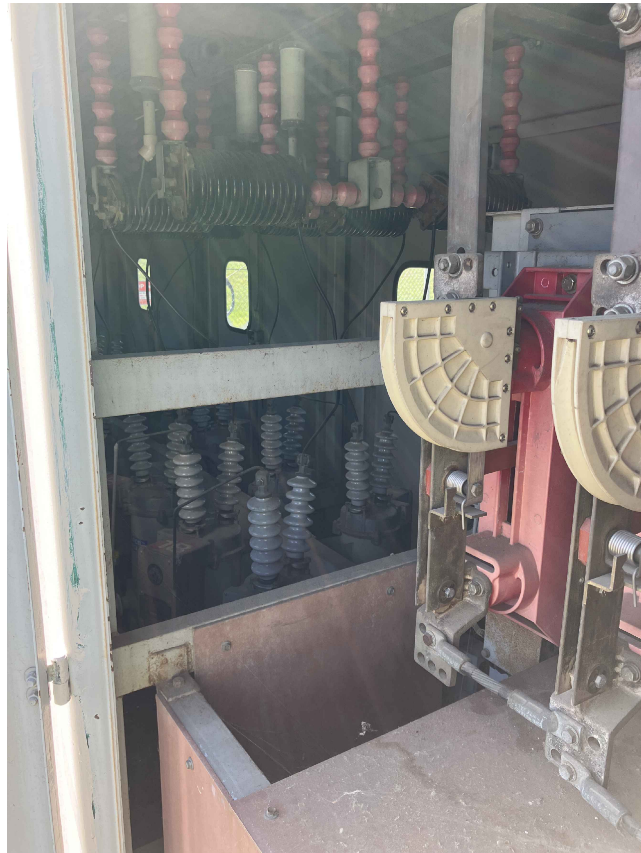
1 EXISTING CAPACITORS SCALE: NONE
