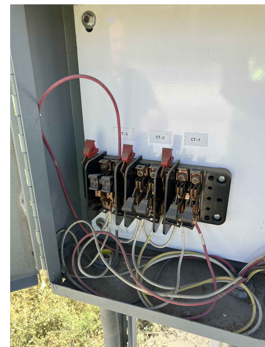
6 EXISTING SWITCH TERMINALS FOR CT'S SCALE: NONE
