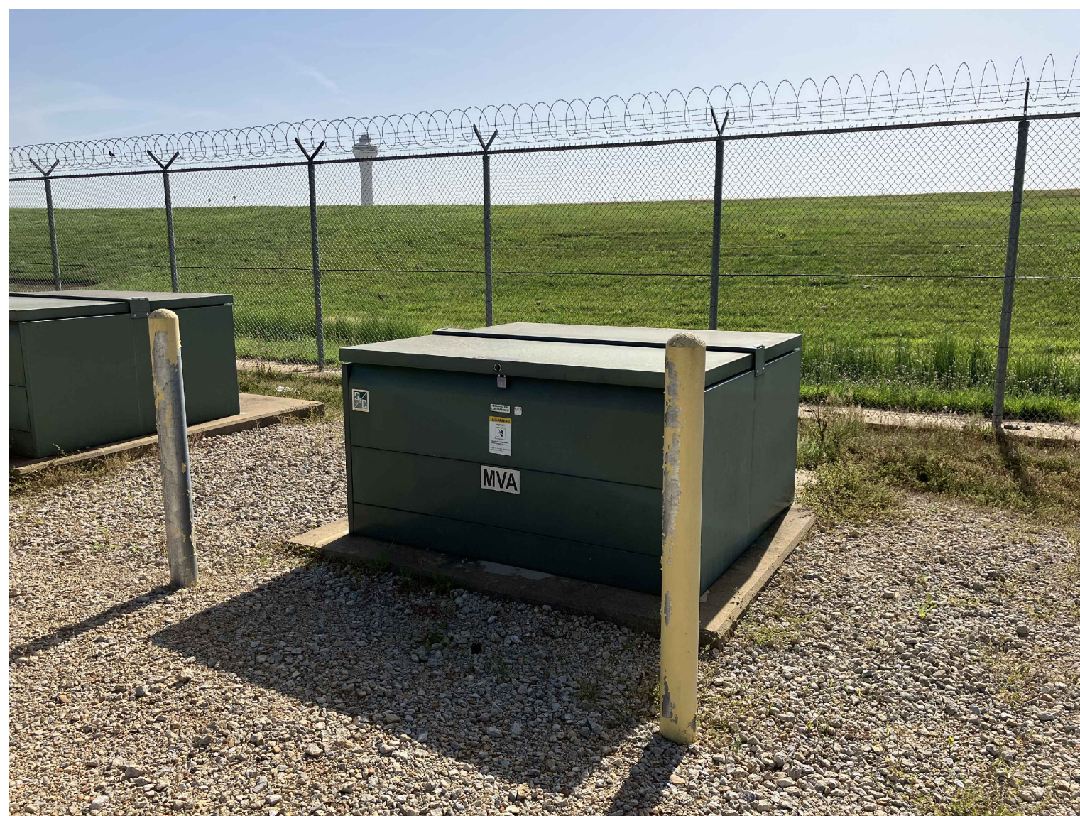
3 EXISTING SWITCHGEAR MVA SCALE: NONE
