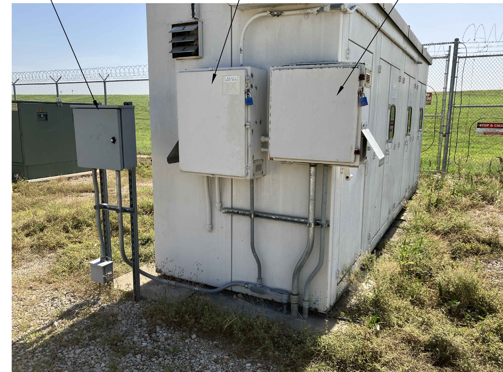
5 EXISTING CONTROLS CABINETS SCALE: NONE
