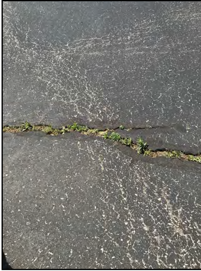
Photo 5 APME-001 Wide Crack
