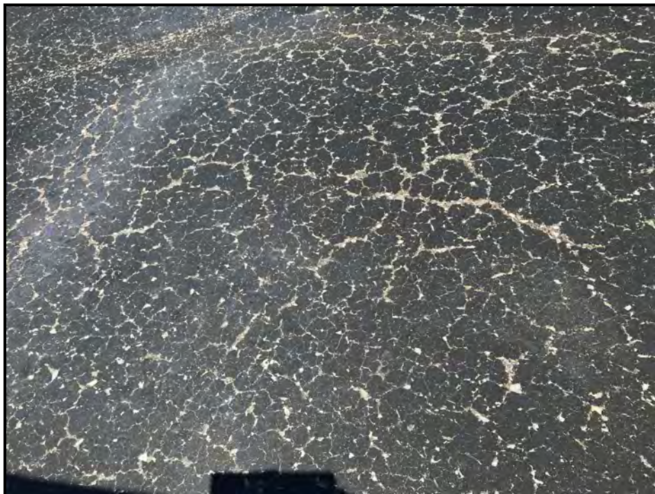
Photo 6 APME-001 Typical Coal Tar Raveling (SE Side)
