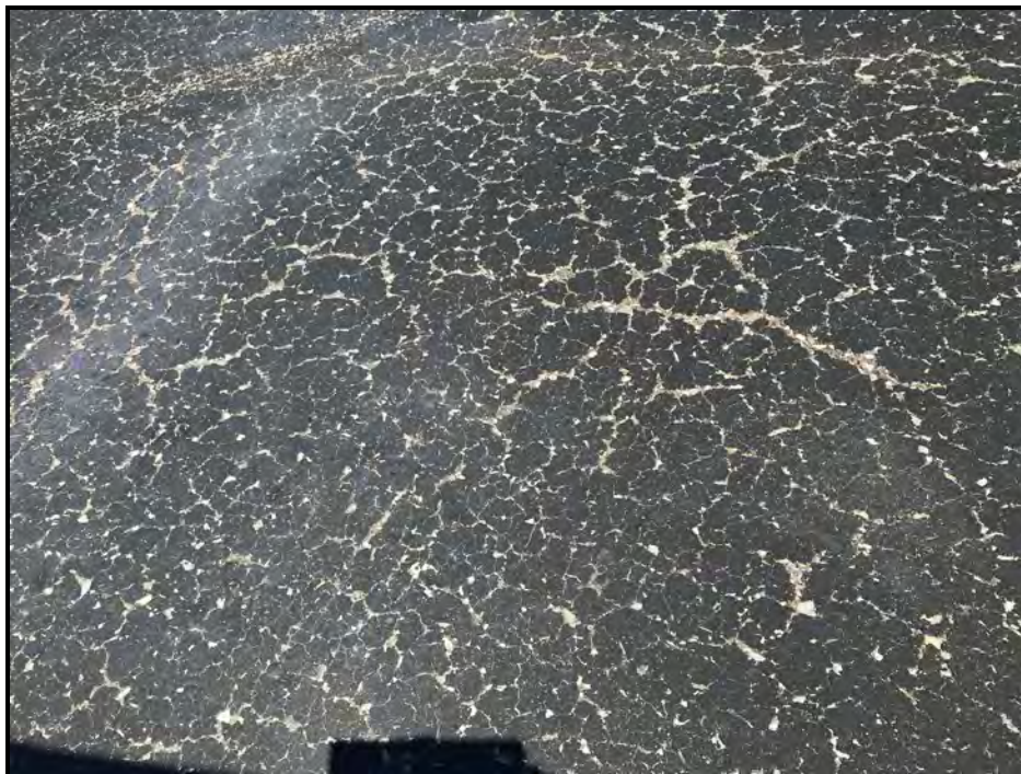
Photo 6 APME-001 Typical Coal Tar Raveling (SE Side)
