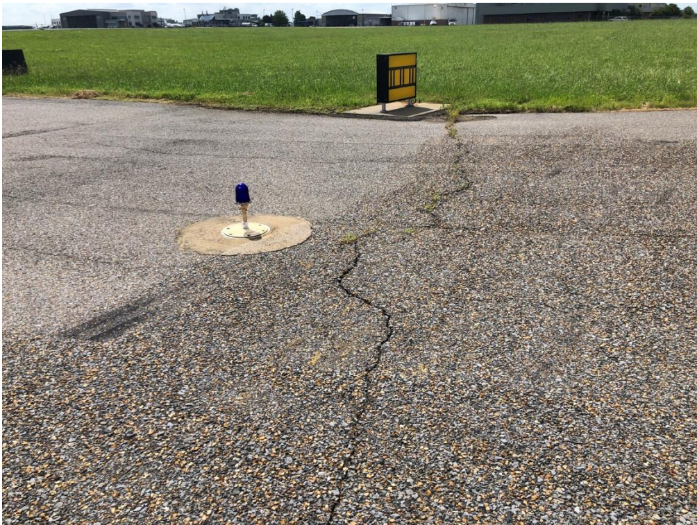
Typical Edge light on shoulder
