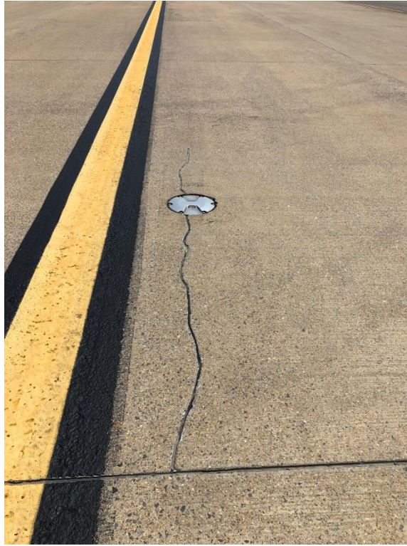
Cracking along Alpha that has been routed and sealed
