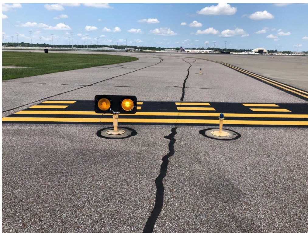
Elevated Runway Guard light and LED Taxiway Edge Light
