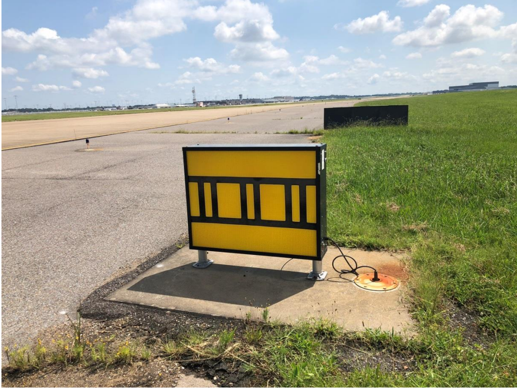
ILS Holding Position Sign @ Taxiway Alpha and November
