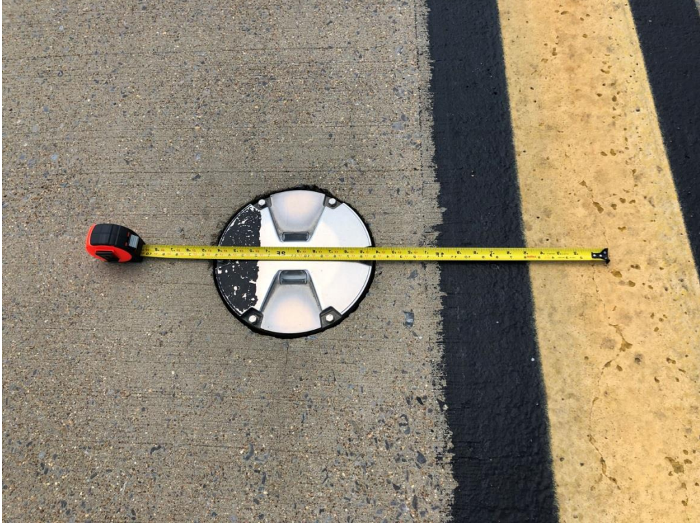
Centerline light along Taxiway Alpha approx..2' from stripe
