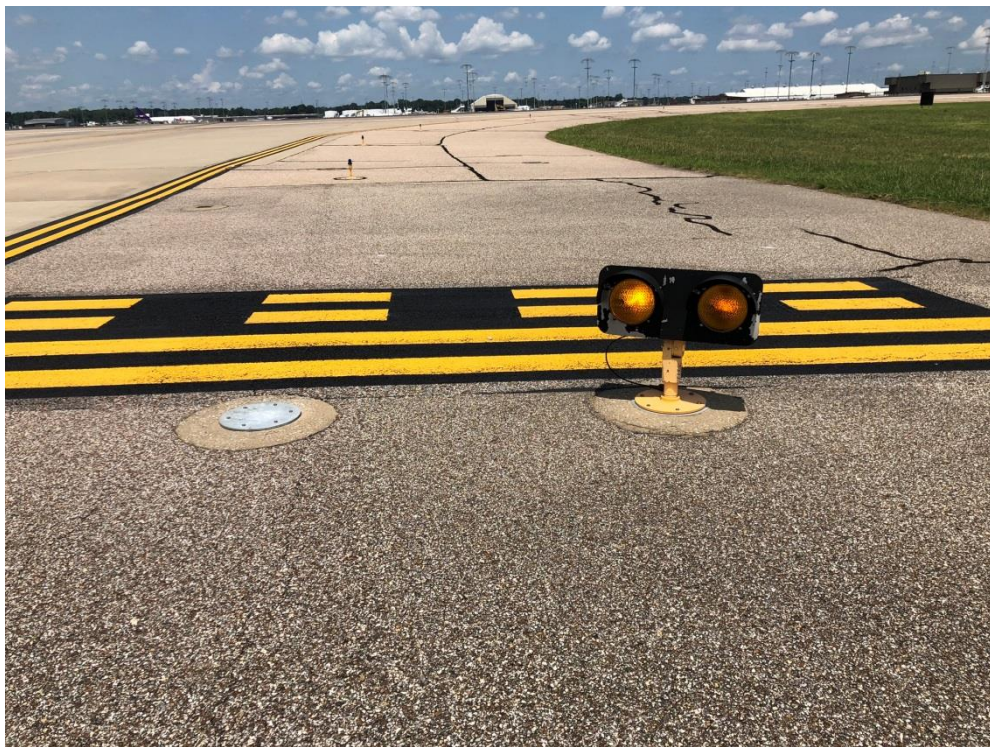
Elevated Runway Guard Light
