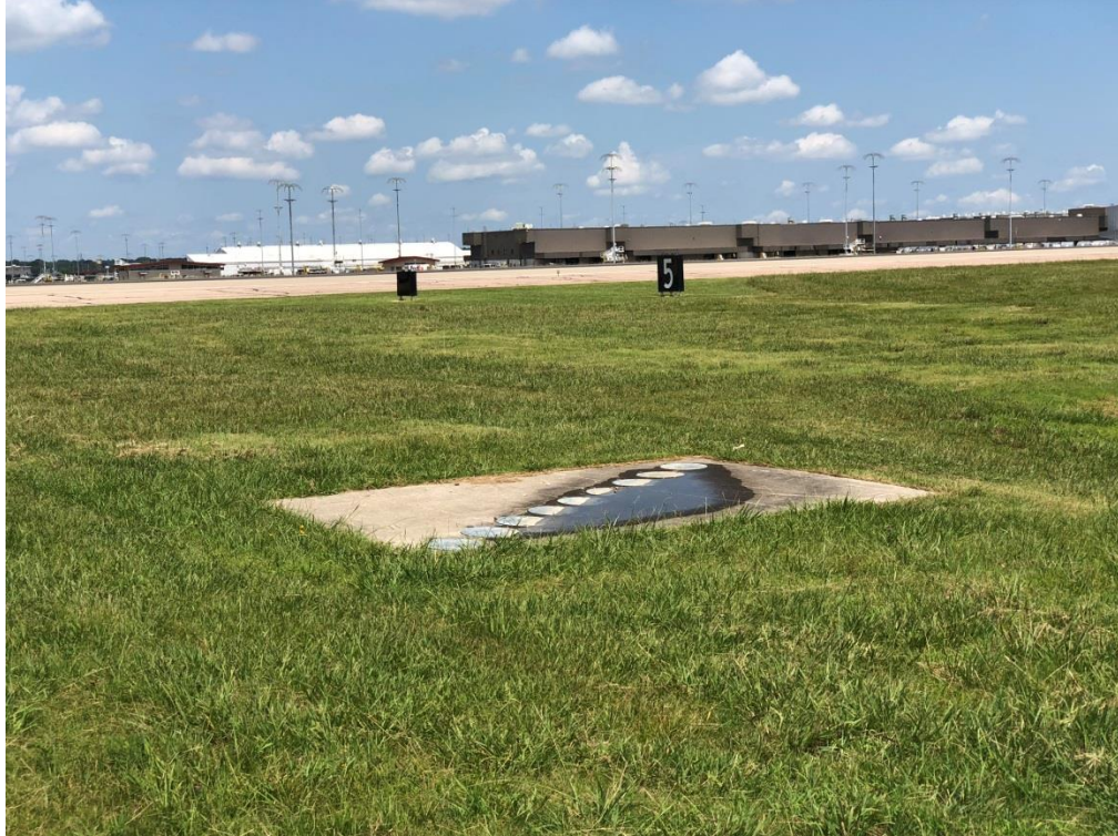
9-Way Can Plaza holding water
