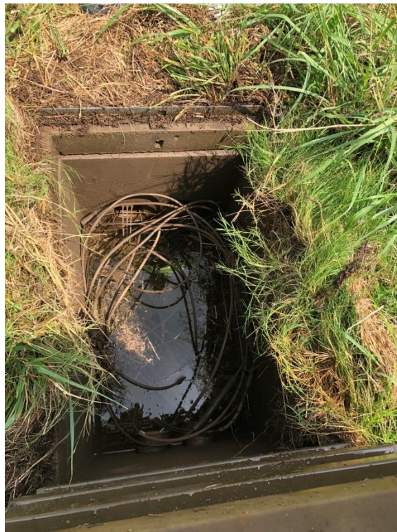
Airfield Electric Handhole
