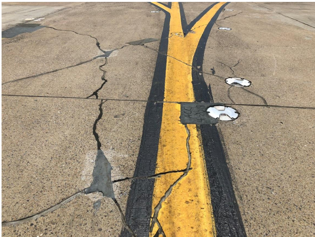
Distressed Area at Taxiway Sierra Centerline north of Taxiway Alpha
