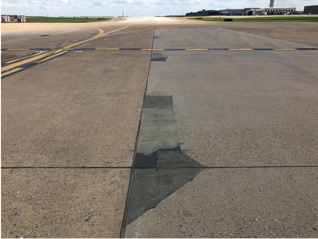
Extensive patching at Taxiway Charlie & Taxiway Alpha Intersection
