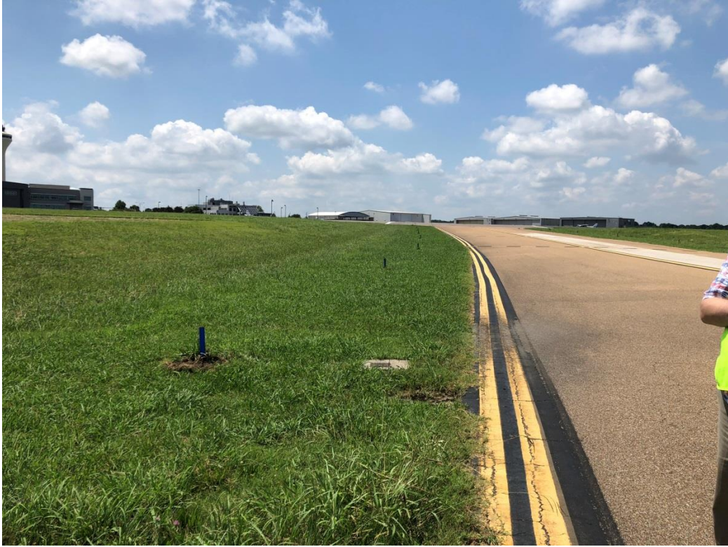
Existing L-853 Blue Taxiway Edge Reflectors along Taxiway X-Ray
