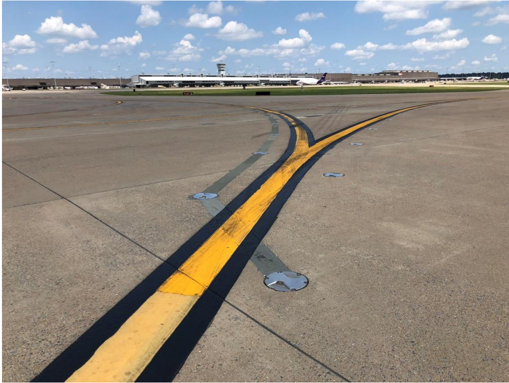
Existing shallow radius “pancake cans” installed at Bravo Intersection
