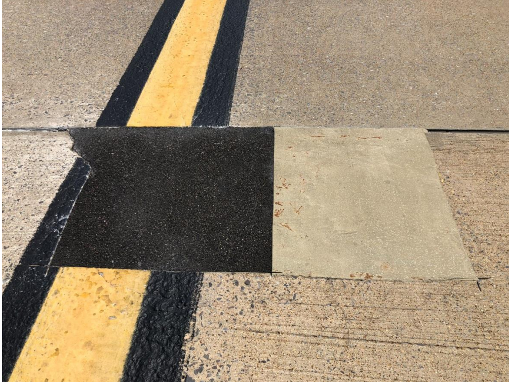
Crack/Edge Repair along centerline
