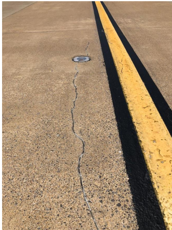
Routed and Sealed longitudinal crack just south of centerline near Charlie
