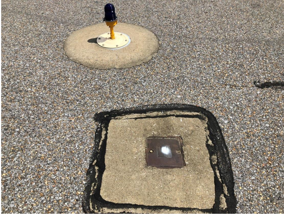
Existing underdrain cleanout (typical)
