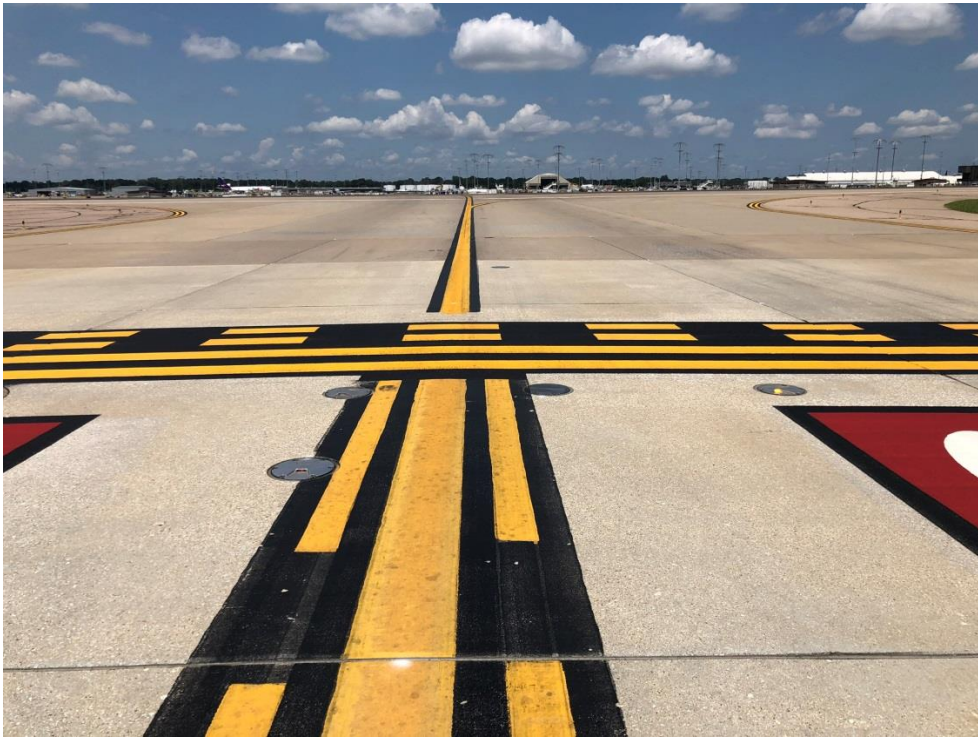
In-pavement Runway Guard Lights @ 9-27 Hold
