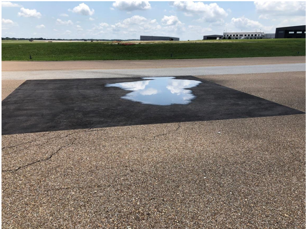
Standing water (bird bath) at existing Taxiway X-Ray/Alpha intersection
