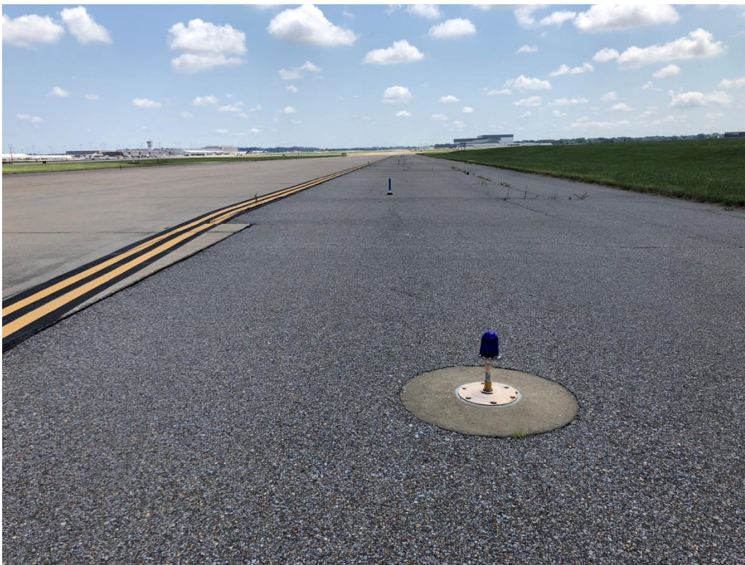
Taxiway Edge Light and L-853 Blue Taxiway Reflector in the distance
