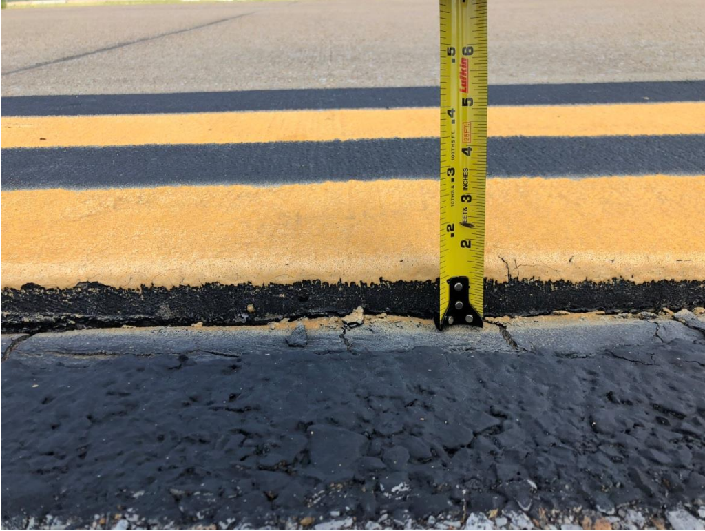
Inch and a half drop off at existing PCC pavement/asphalt shoulder interface
