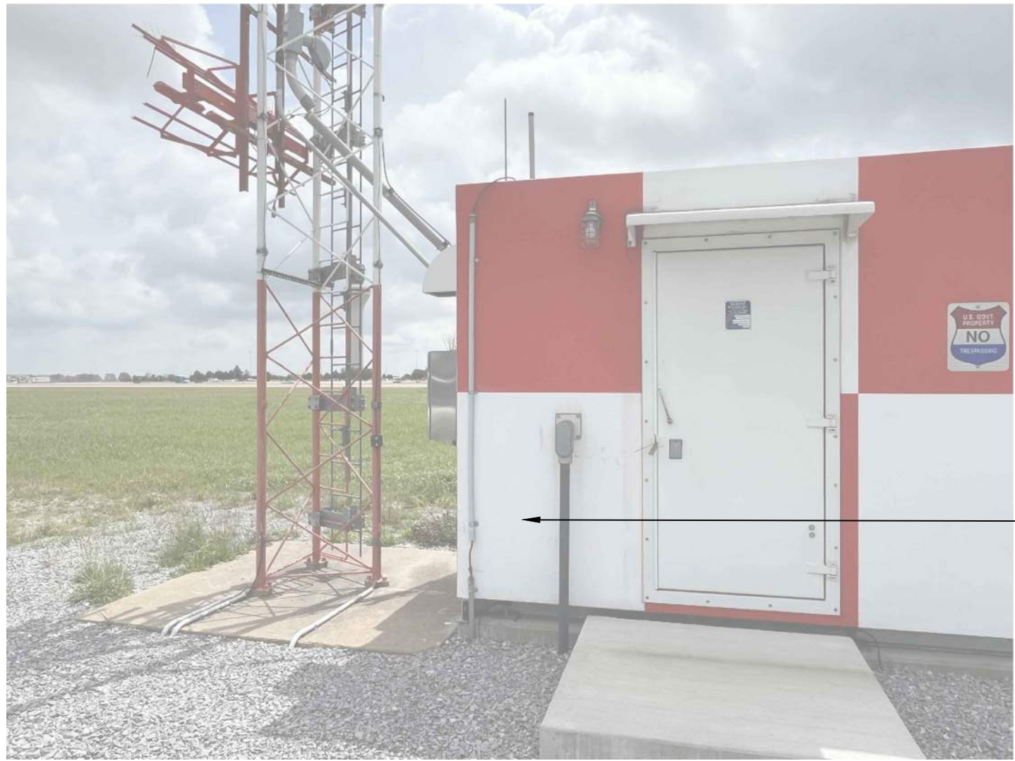
2 CONDUIT CONNECTION LOCATION PHOTO SCALE: NONE
